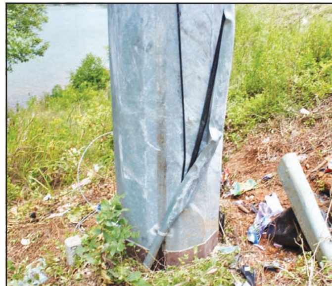
A Hayesville man died after crashing his vehicle into this concrete power pole off US 76 on Saturday, Aug. 3.
